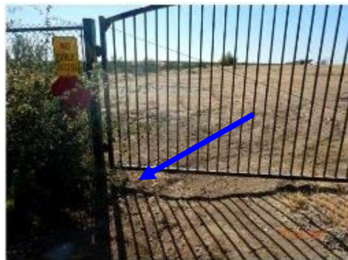
MIP Figure 2.0.A - Outfall 1
